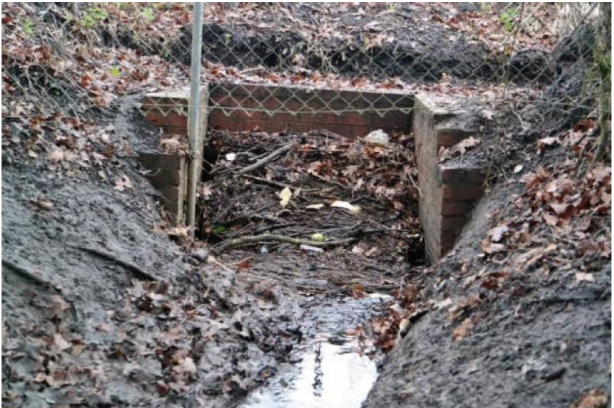
Figure 4-6 The blocked culvert entrance on Cuddington recreation ground. Source: Resident
