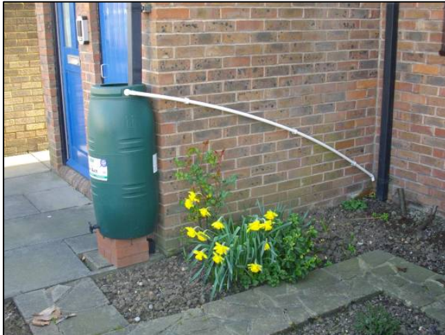
Figure 4-7 Example of a 100L Water Butt retrofitted to existing development
