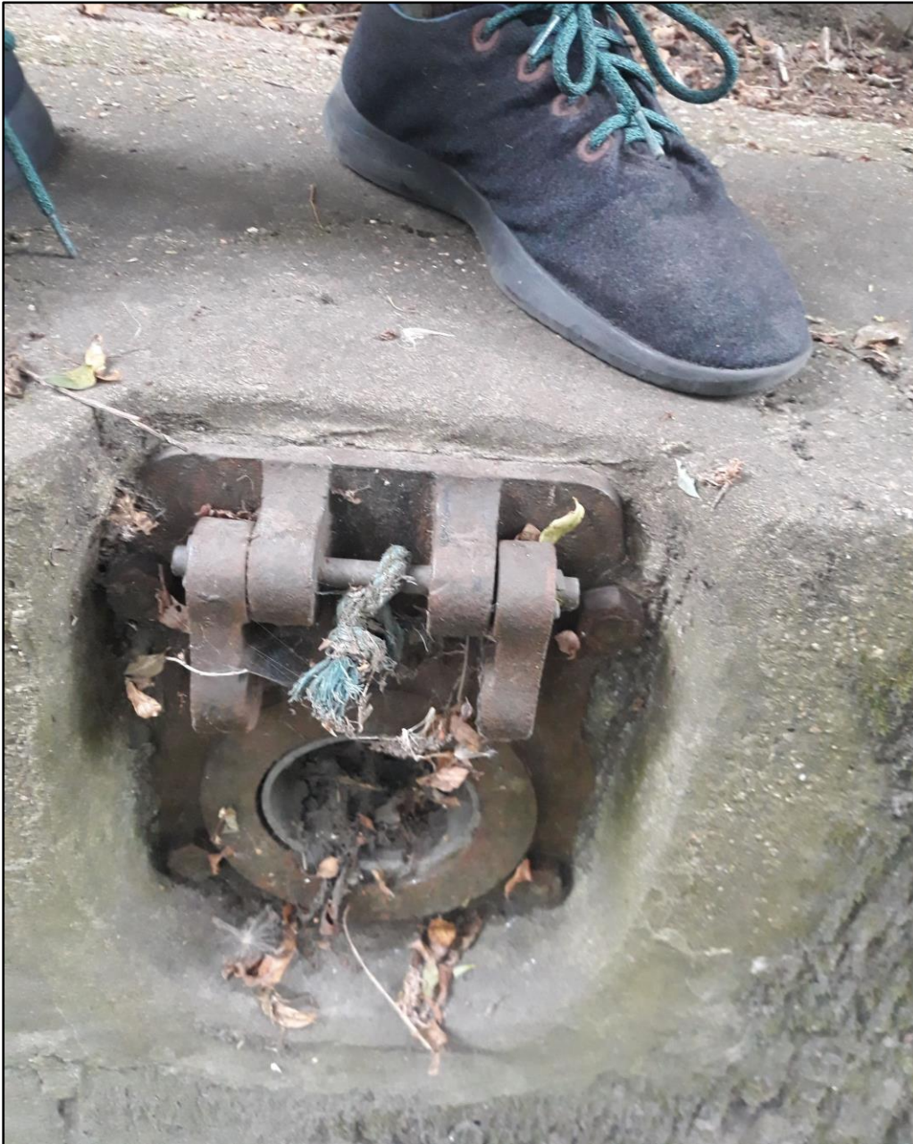
Figure 2.2. Broken Flap Valve
